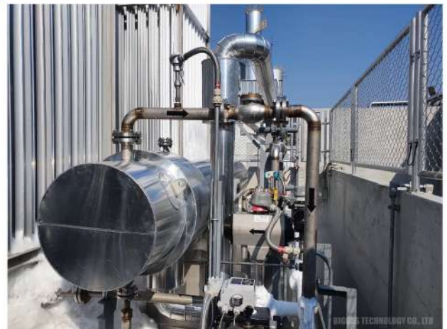
Heat Recovery System
